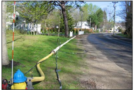
By installing temporary lines like this 6" PVC pipe on Brown Street in Kennebunk, the District is able to replace its obsolete 1930s era pipe with a new one in the same location, minimizing the impact on both customers and other underground utilities.
