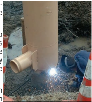
District Facilities Technician Gerry Goulden welds the pitless adaptor onto the 18" steel casing at the Merriland River well site.
