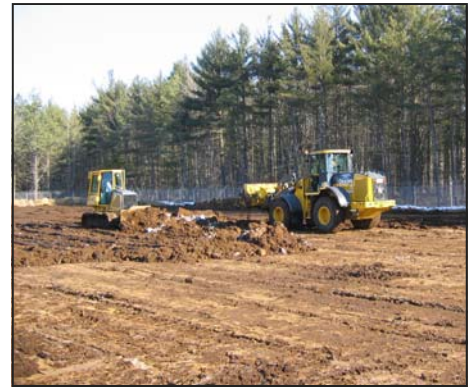
Step 3. During the winter, "sludge" is removed from the lagoon and spread 3" thick on the drying bed to be freeze-dried.
