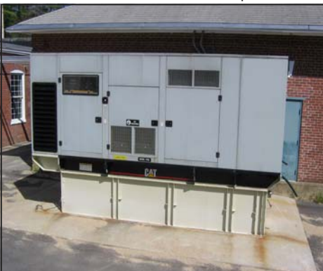
"Papa Bear" - is our largest 800 kW standby diesel generator that runs the Treatment Plant during power outages to produce up to 6 mgd.
