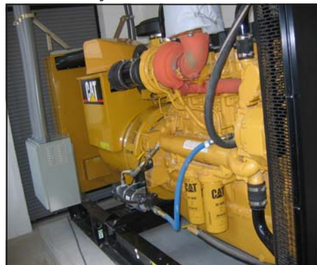
"Mama Bear" - refers to our 350 kW standby diesel generator that runs the PTR facility, producing up to 3 mgd of treated well water.
