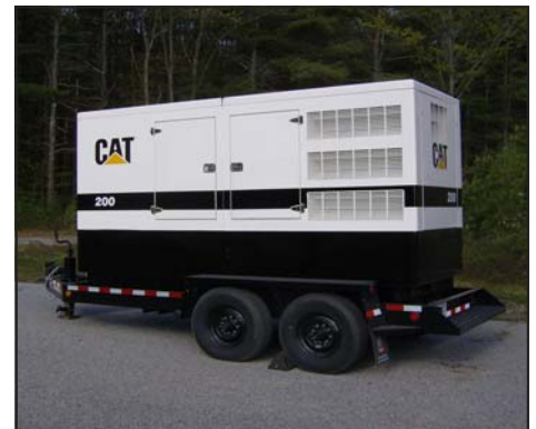
"Baby Bear" - this ultra quiet 200 kW portable diesel generator can be towed to any District facility as needed when the power goes out.
