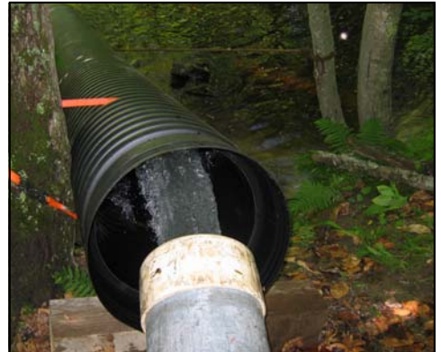
An initial flow test yielded around 1.8 MGD of high quality water. Following the "break-in" period, flows over 2 MGD could be realized.
