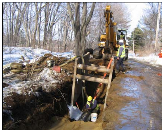
District crews got off to a cold and early start in February '08, installing over 650' of 16" diameter main in Cape Porpoise (Kennebunkport) to improve water supply capacity.
