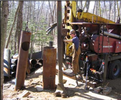
Drillers install an 18-inch diameter gravel well to back up the existing 12-inch diameter production well at the District's Merriland River Well site.
