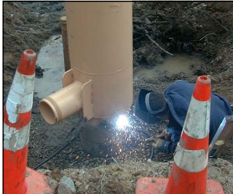
Sparks fly as the District's Gerry Goulden welds a pitless adapter onto the 18-inch diameter steel casing. Precise vertical alignment is critical.
