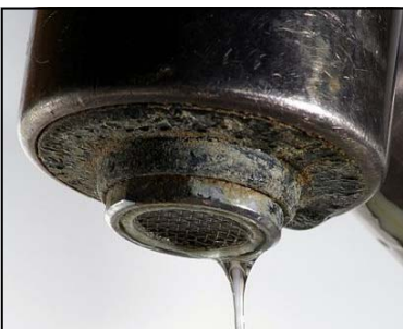
The scale on this hot water faucet is readily removed with any commercial grade calcium-lime-rust type cleaner.
