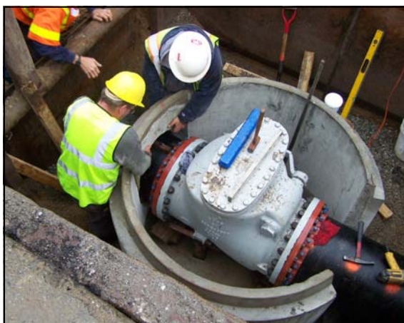
Crews install a large 20" diameter check valve as part of the $800K Route 1 main replacement project in Wells. The check valve is used to separate pressure zones.
